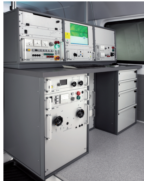
IRG 3000, integrated in the cable test van
